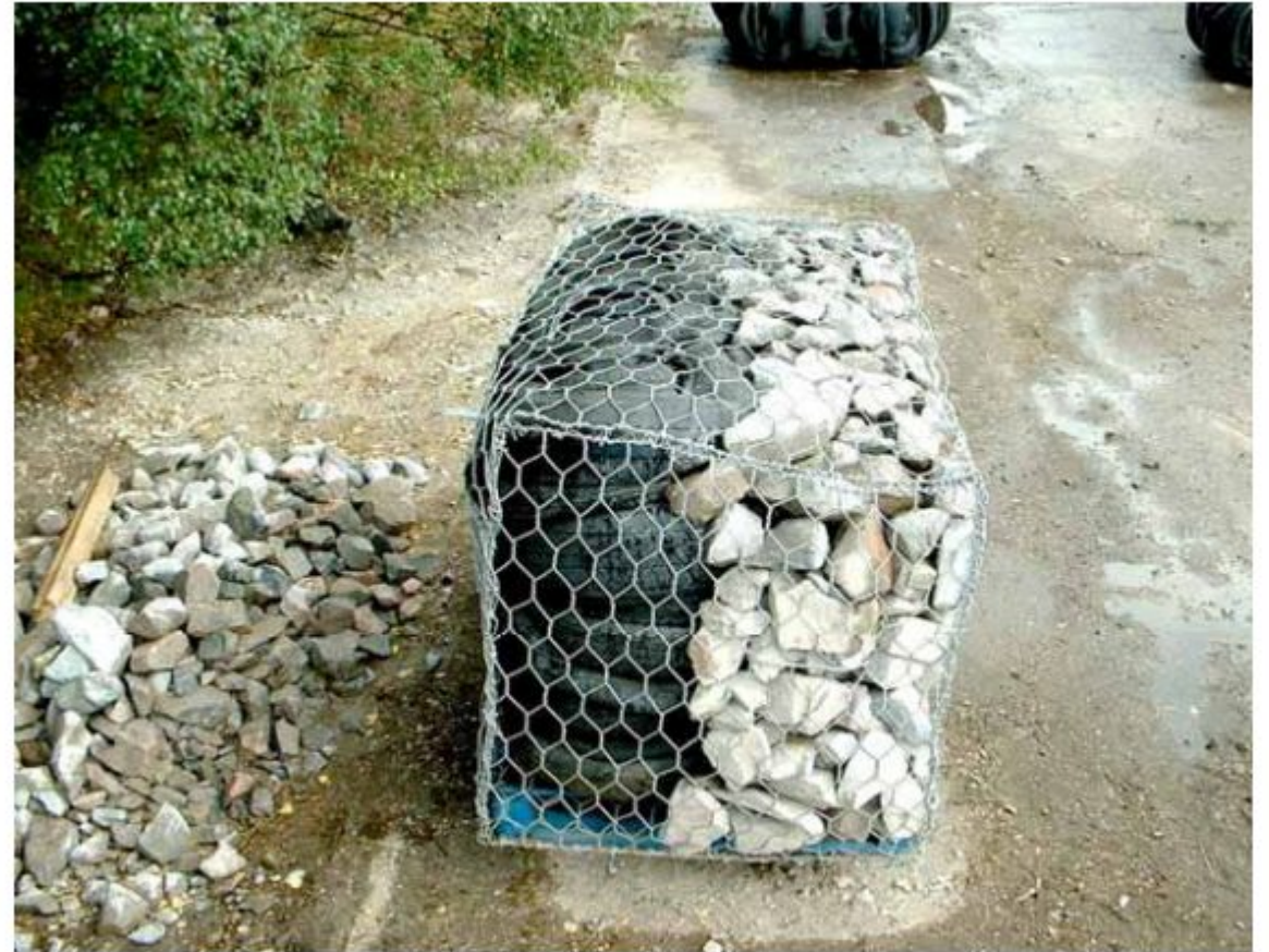
Figure 5.39 Tyre bale as rear fill for gabion box (courtesy Northern Tyre Recycling)
